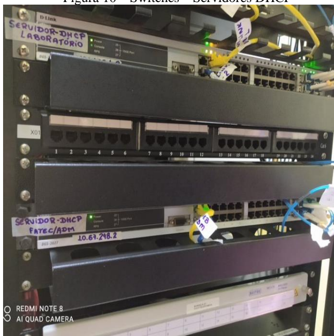
Figura 10 – Switches – Servidores DHCP
