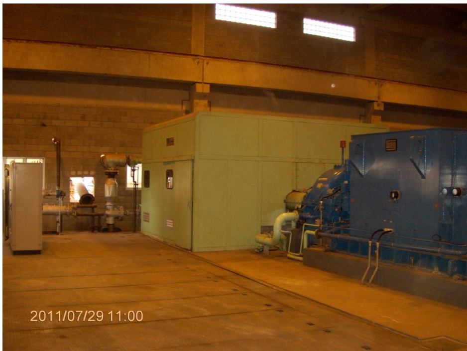
Figura 17 - Turbina e painel (AMARAL, 2012)
