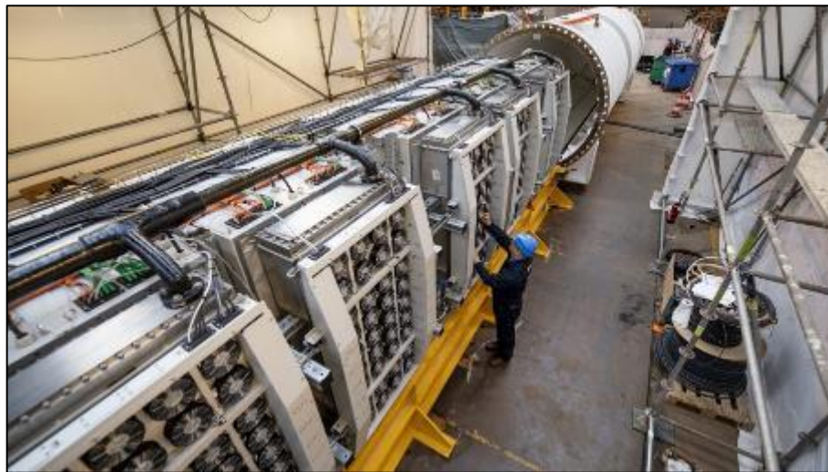
Figura 16: Data Center submerso Microsoft
